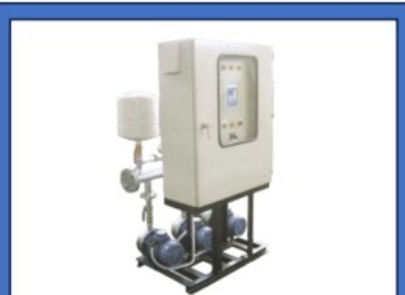
VARIABLE SPEED BOOSTER PUMP
